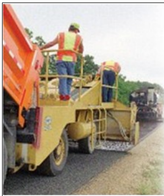
Chip seal is a fundamental pavement preservation process, here placed in Minnesota.
