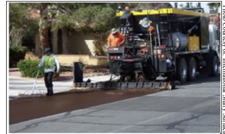
Unit of American Asphalt and Grading Company places slurry seal as part of year-long work with the City of Las Vegas in 2009.
